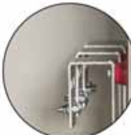
Incoming power terminals
