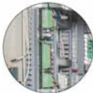
Control I/O terminals
